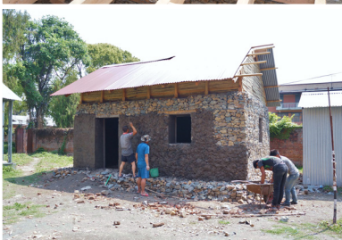
Picture: Demonstration Unit - Pulchowk Engineering campus, Kathmandu, Nepal ©A&D
