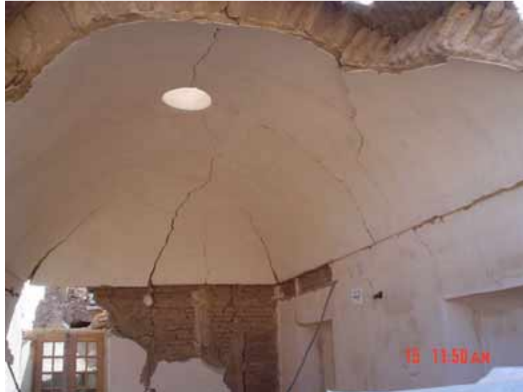
Figure 8: A barrel vault with cracks in Arg-e-Bam
