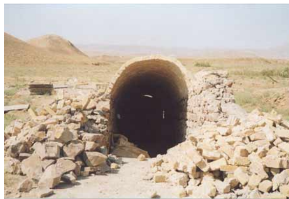
Figure 4: A masonry barrel vault, 3 km from Avaj's fault, western Iran
